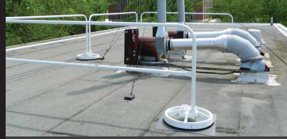
HVAC / ROOFTOP EQUIPMENT
