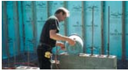
Pouring in the dry cement mix along with water from a hose
